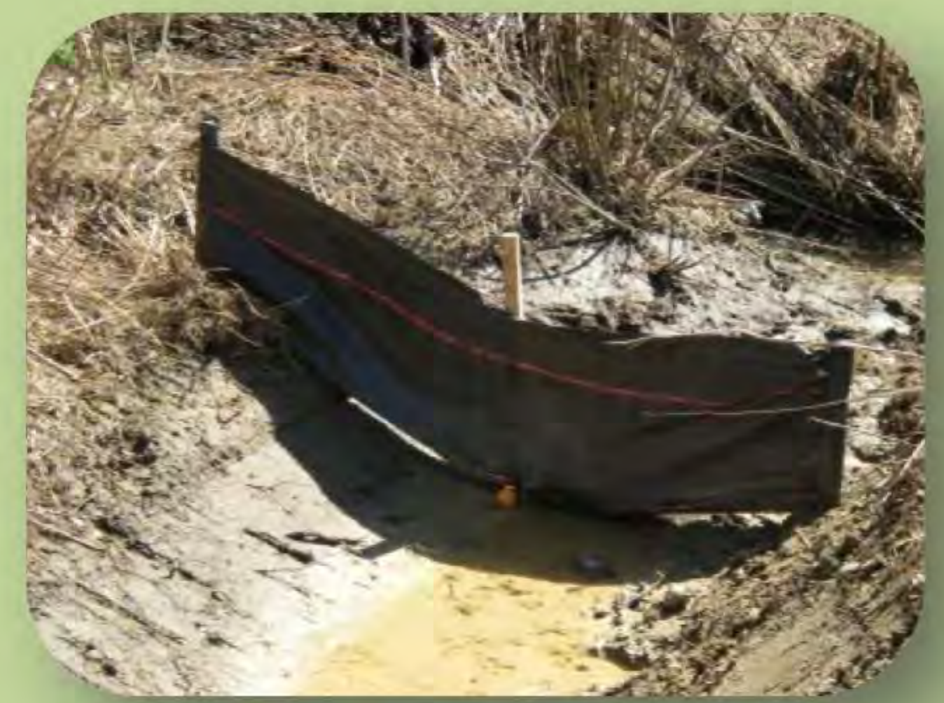
WRONG! An example of an ineffective erosion control practice – silt fencing should be buried to a depth of about 8 inches
