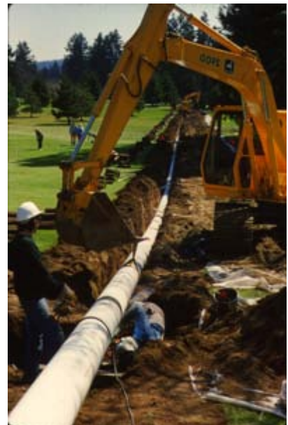
Installing a small diameter distribution pipe; Photo from Naturaas.org, courtesy of Duke Energy Gas Transmission, Canada
