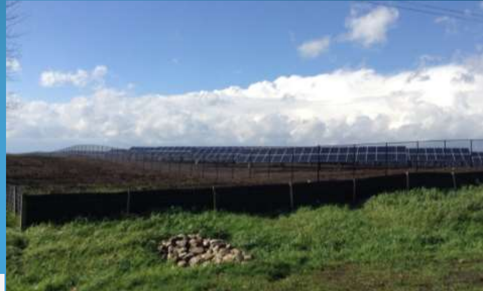
Clarkson Solar Array, Town of Potsdam
