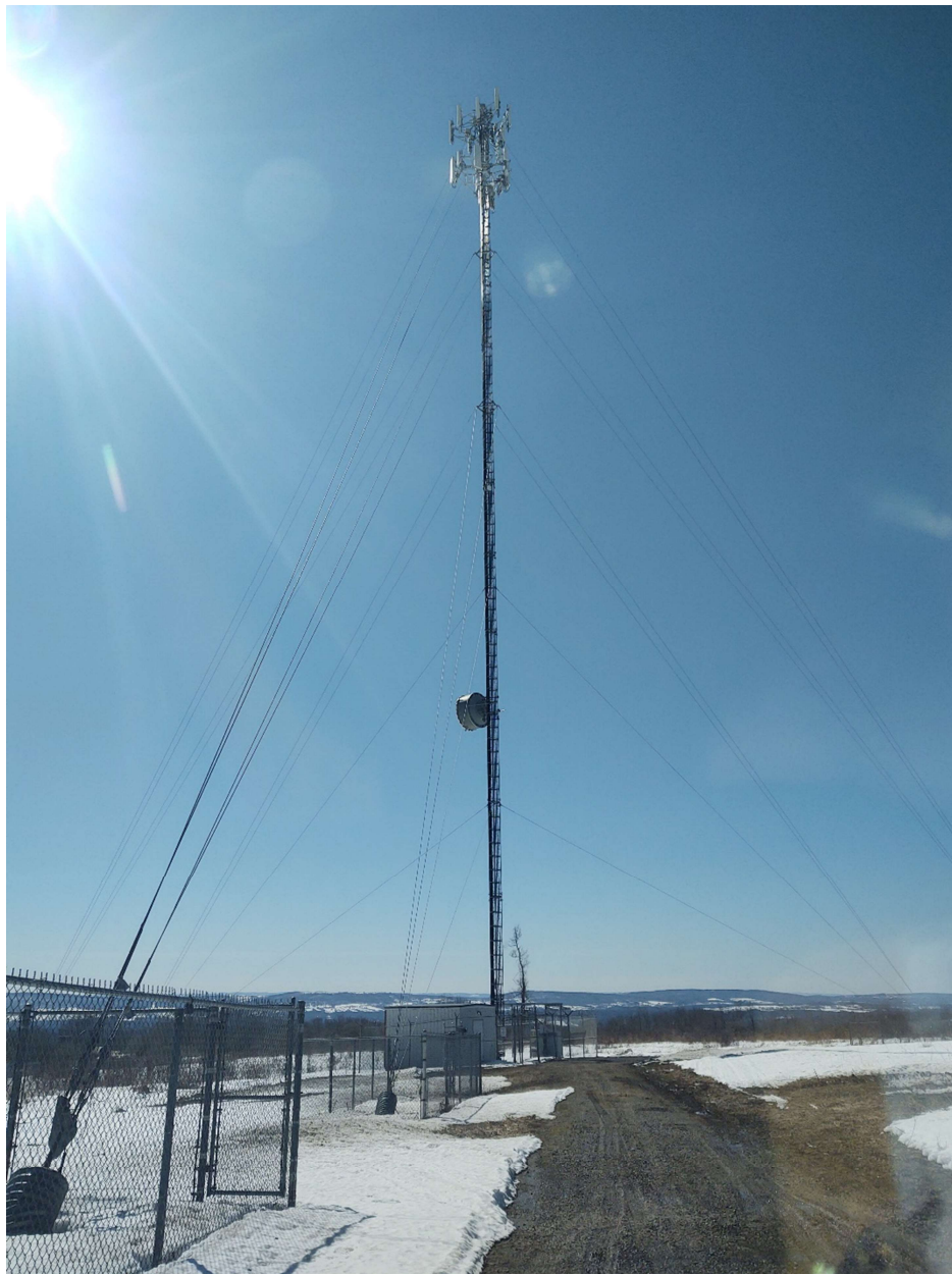
Figure 13 Guyed Lattice Pole Tower
