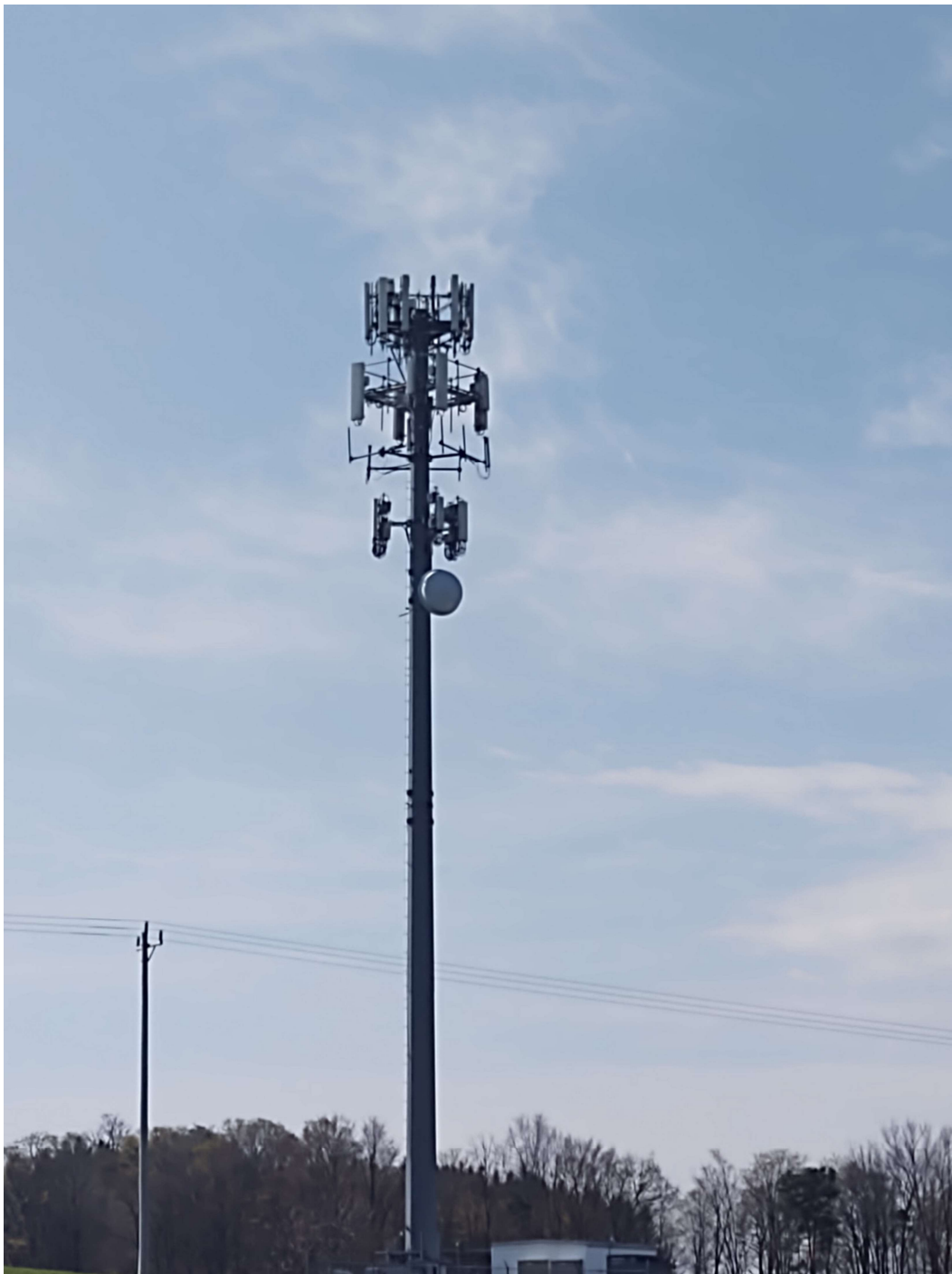
Figure 31 Monopole Tower in Oneida County
